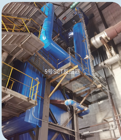
SCR Reactor no. 5
