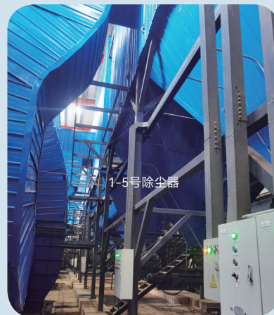
Dust Removal Equipment no. 1-5
