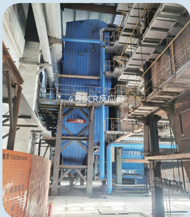
SCR Reactor no. 4
